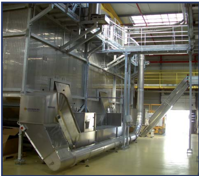
View of bottle pickup at exit of storage silo
